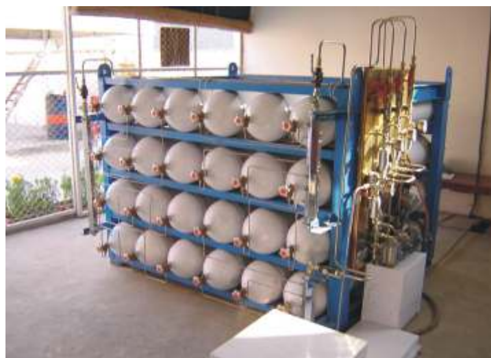
CNG Storage Cylinders Manifold
