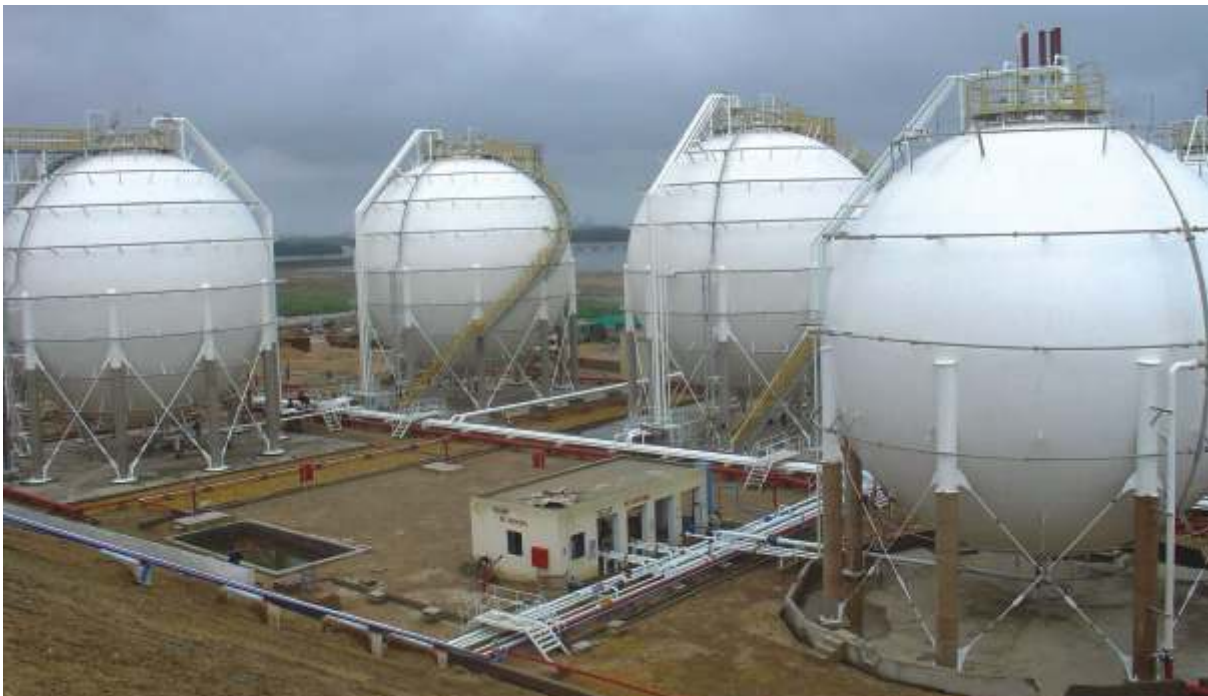
A view of the LPG tank farm area with 3 x 1500 MT and 2 x 1000 MT tanks ready
